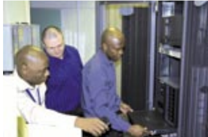
Teamwork ... Romanus Dindi, project manager, with BCX server hardware engineers Clifford Hutton and Anele Meltafa.
