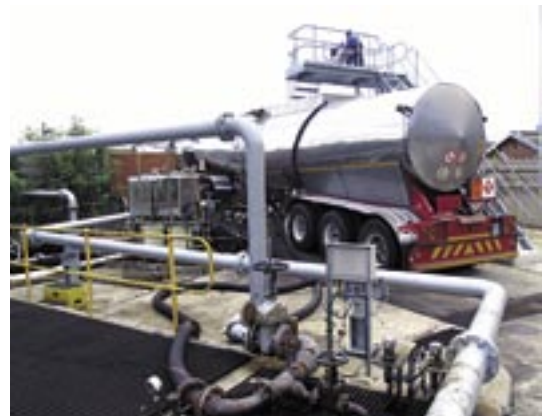
The road-tanker loading facility at Island View.
